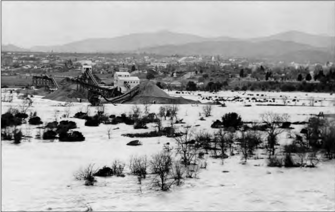
Photo 2: Telephoto panorama of the Redding aggregate processing plant and the Sacramento River crossing of the Redding-Coram belt conveyor as seen from the bluffs to the north of the river (Meriam Library Special Collections Department Shasta Dam Digital Collection, CSU Chico, SC22260, Feb. 28. 1940)
